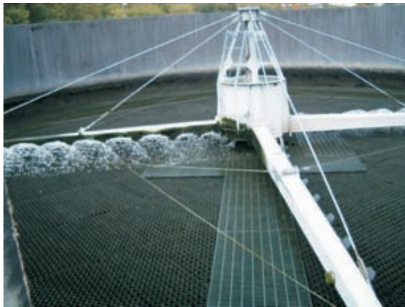
Secondary Treatment Trickling Filter, City of Port Angeles.
